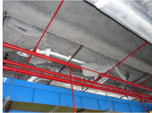
Photo #1900520. Collapsing overhead thermal insulation.
