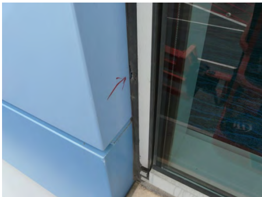
Photo #1910144. Secondary jamb sealant failure.
