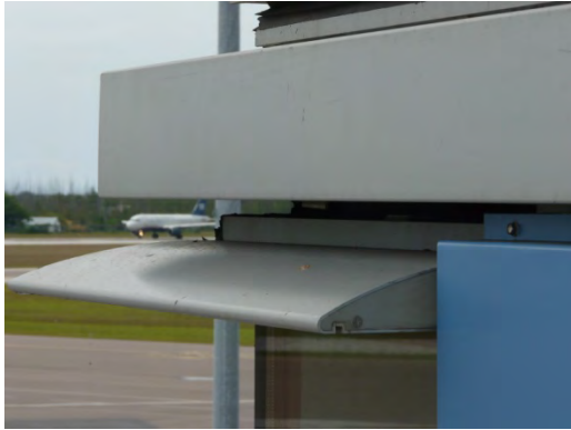
Photo #1910365. Missing primary sealant joint at curtain wall head.
