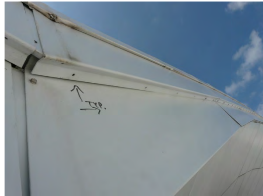
Photo #1930858. Roof fascia panel missing fasteners.
