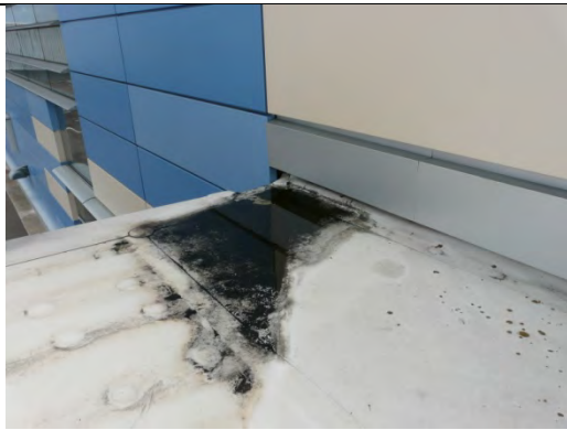
Photo #1910090. Standing water on roof. Water discharging into wall.
