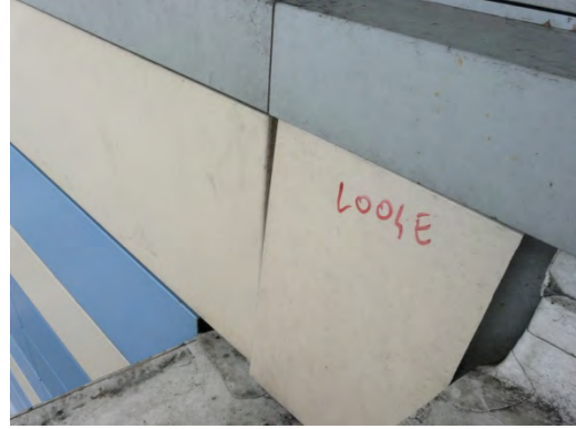
Photo #191001. Wall panel visibly misaligned and showing excessive deflection when touched by hand.
