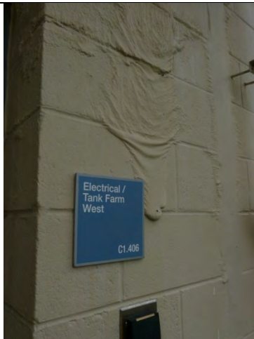
Photo #1920765. Blistering of elastomeric coating.
