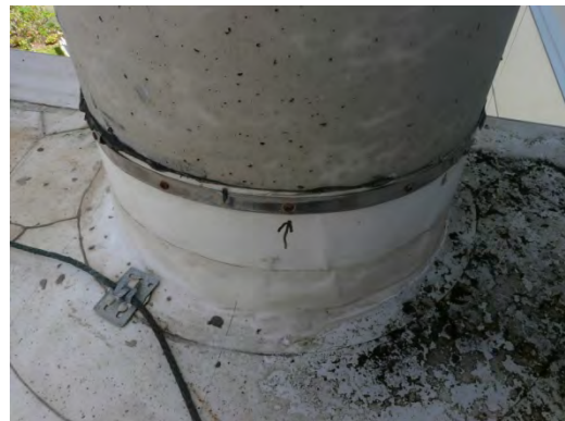
Photo #193051. Unsealed roofing termination.
