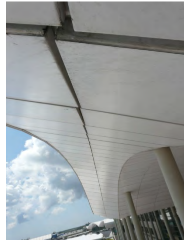
Photo #193044. Soffit panels visibly misaligned.
