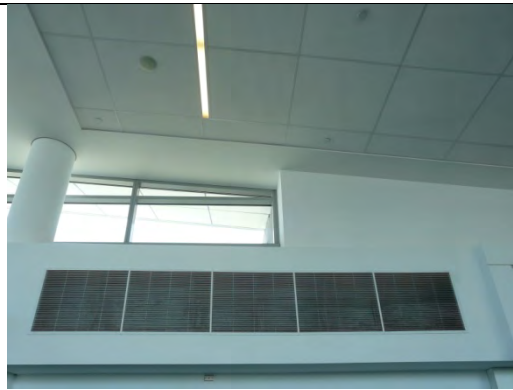
Photo #1930329. Leak above soda machine near [REDACTED].
