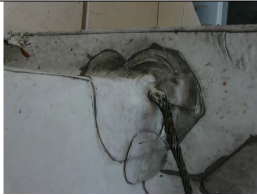
Photo #1900075. Improperly detailed, unsealed roofing termination.
