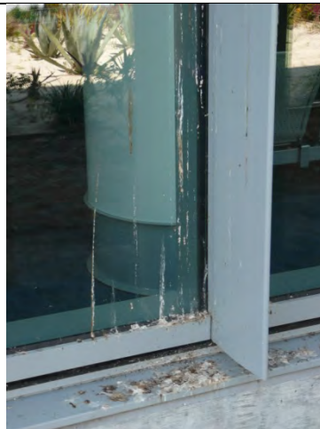
Photo #1890415. Bird deposits on a curtain wall near the rest area.
