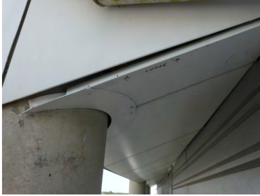
Photo #1930508. Soffit panel visibly sagging and showing excessive deflection when touched by hand.
