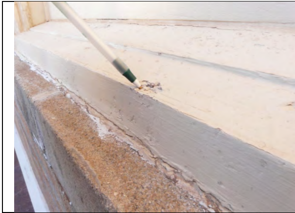
5. One of the deepest observed dents at the window sills, resulting from a hailstone impact . Window #99, 12/18/2014
