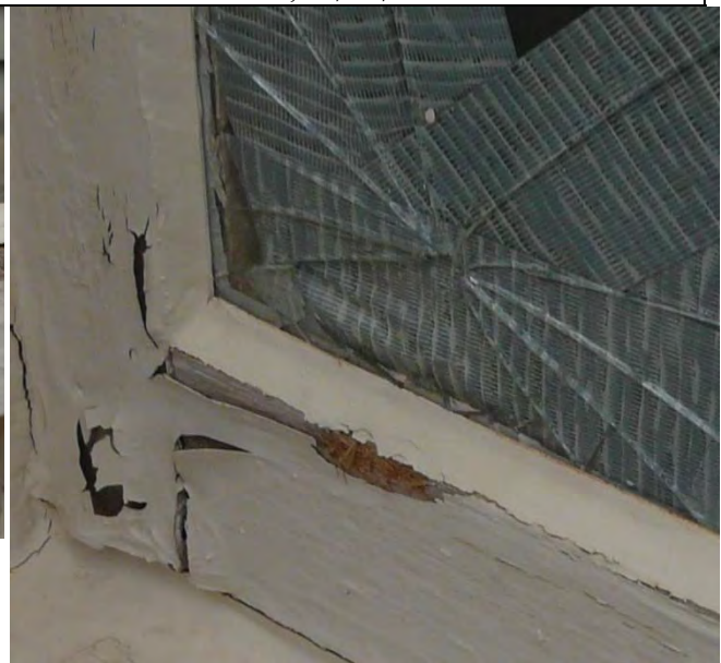
4. Close up of the photo reproduced above, focusing on the bottom rail damage. Window #65, 12/17/2014
