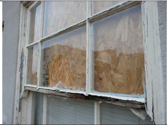
6. Glass breakage of an upper sash, with glass panes deadloaded on a rotten meeting rail. Wood rot and loss of coating are preexisting conditions. However, this member may need to be restored in order to reglaze the window. Window #5, 12/17/2014
