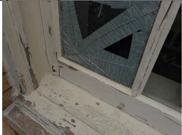
2. Typical impact signature to the bottom rail and glass, resulting in simultaneous direct impact breakage of glass pane and indentation of wood, which gives an idea of the size of the hailstone. Also, the indentation of the wooden sill and its coating is visible below. The peeling coating is a preexisting condition. Window #65, 12/17/2014
